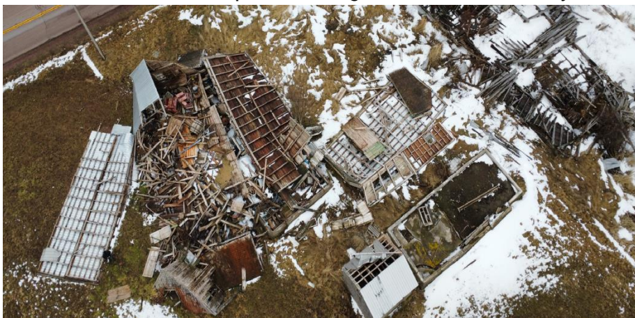
Hurricane Fiona damage to barn.
